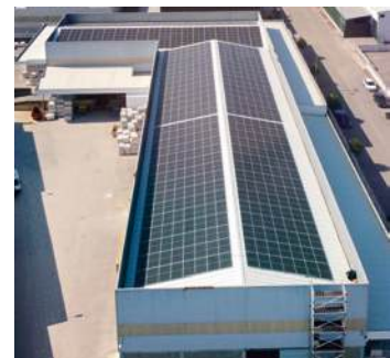
TopCer 2 warehouses, are covered by 1036 photovoltaic solar panels
